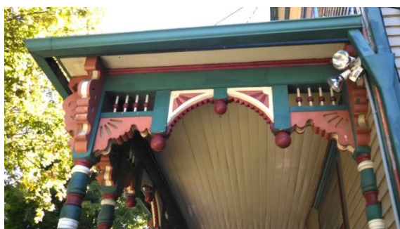
Figure 2: Highly decorative detailing of the porch of the Mumaw House shows typical detail of a Queen Anne home, c. 1890s, photo by Cara Maib ©2014
