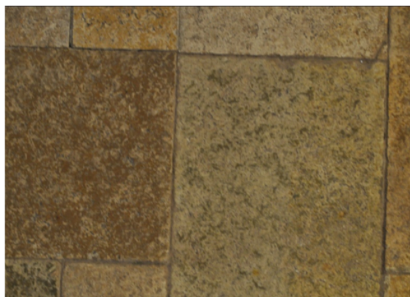
Figure 10: The interior of the Maynard-Campbell House still has its original floor tiles composed of sawdust and cement. Photograph by Nick Hullibarger.
