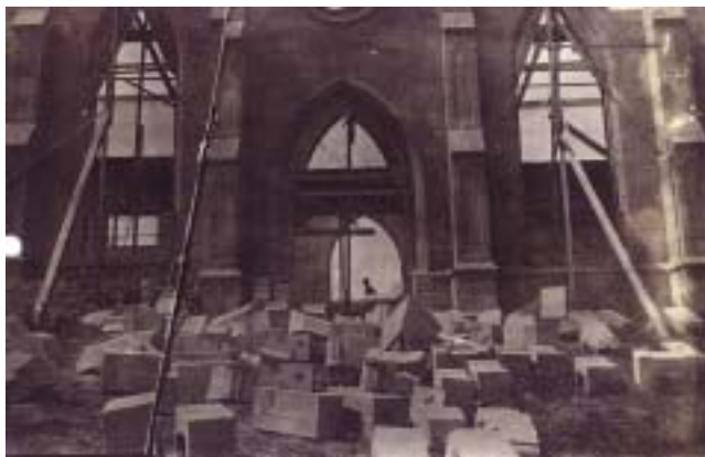
In 1905, the construction began. Pictured are the bricks and stones that were used.
